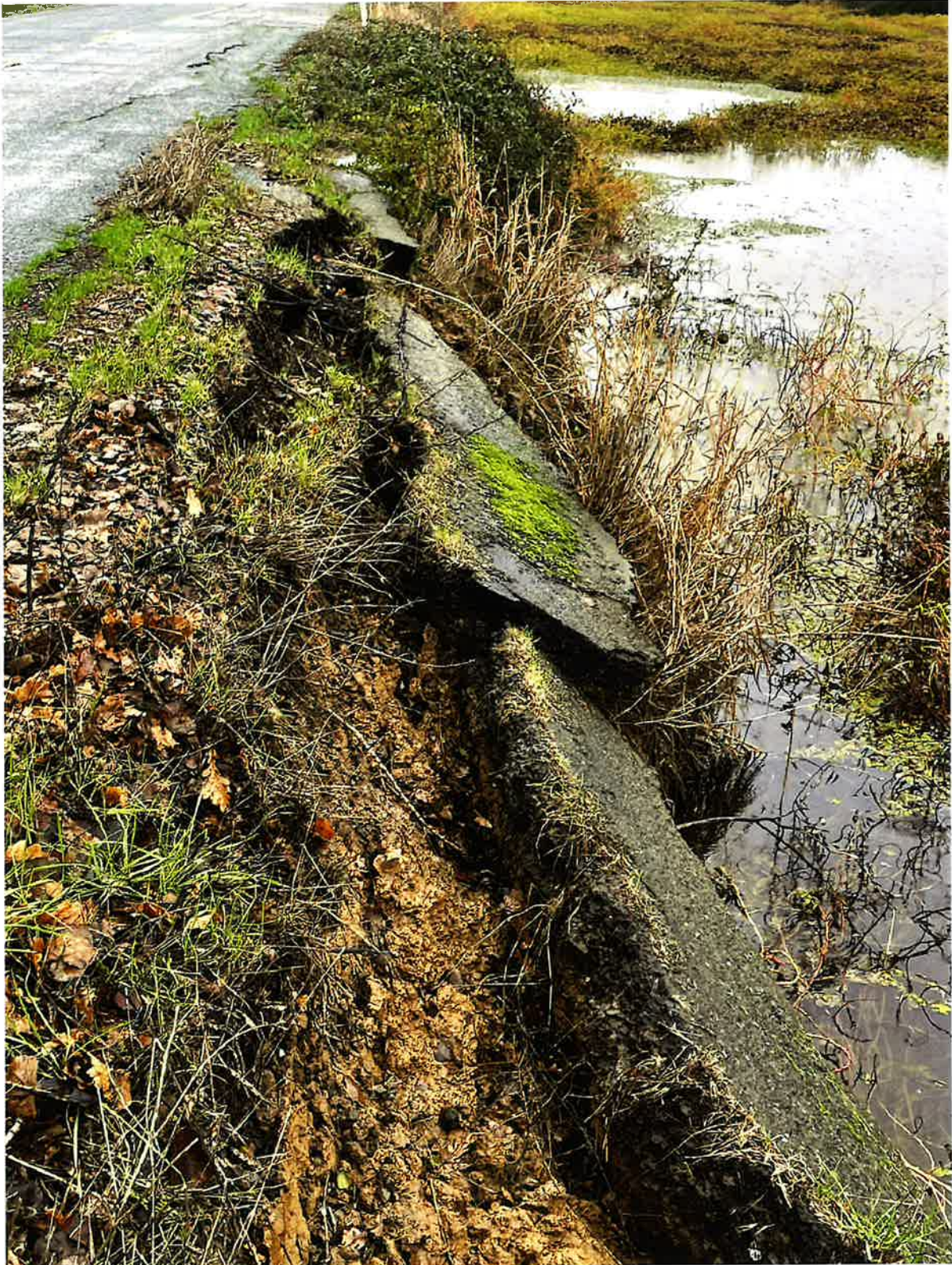
PHOTO 4: PREVIOUSLY REPAIRED SITE PRE-REPAIR CONDITION
