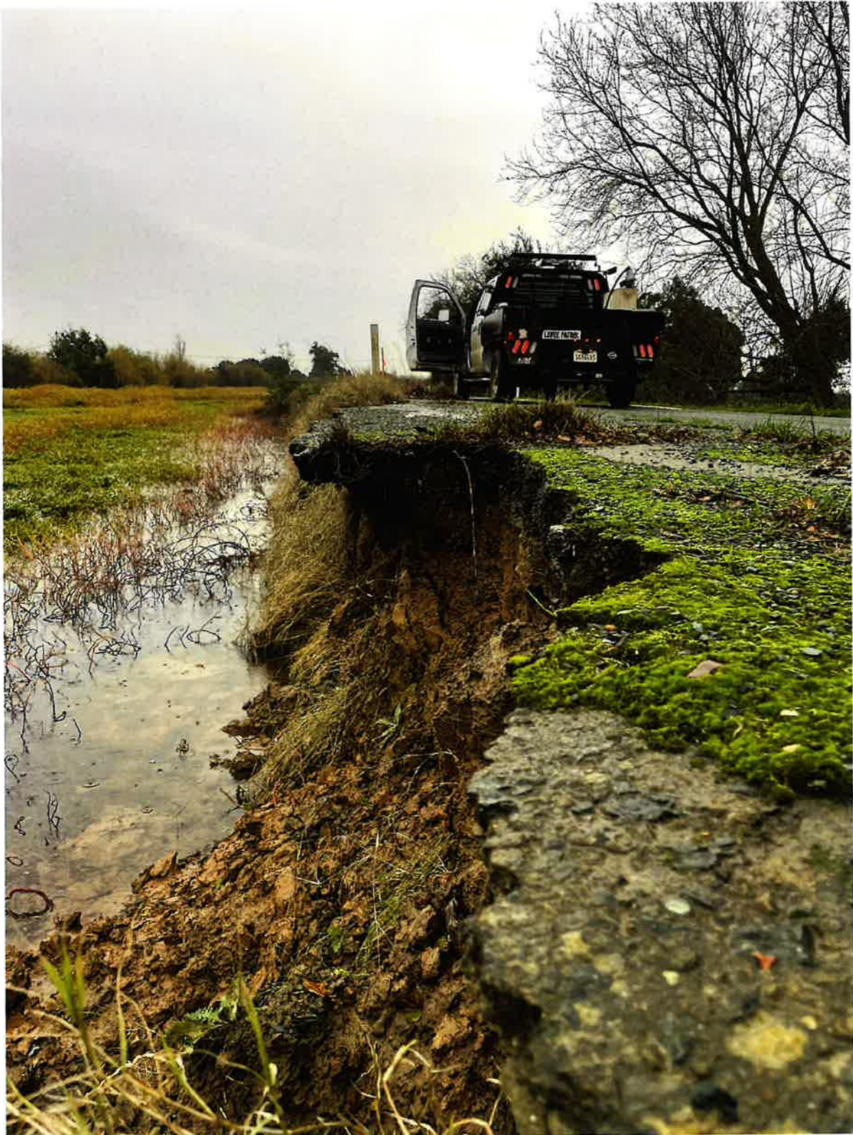
PHOTO 3: PREVIOUSLY REPAIRED SITE PRE-REPAIR CONDITION
